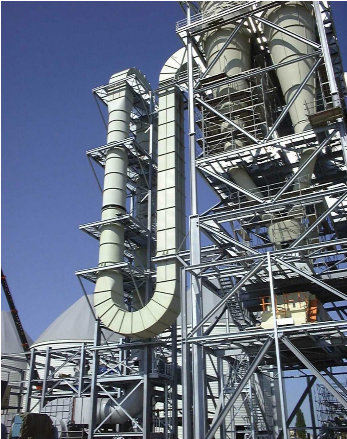
loop framework next to the dryer cyclones (TR)
